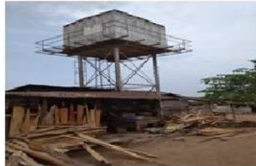
PLATE 6: ABADONED OVER HEAD TANK OF BORE HOLE WATER AT ILUPEJU IJAN
