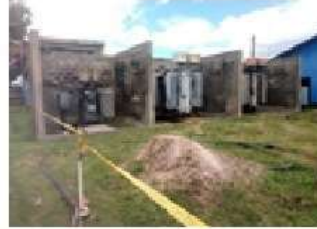
PLATE 2: ABADONED POWER TRANSFORMER AT ERO DAM
