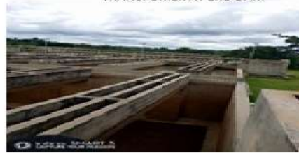
PLATE 4; ABADONED WATER FACILITY AT ERO DAM
