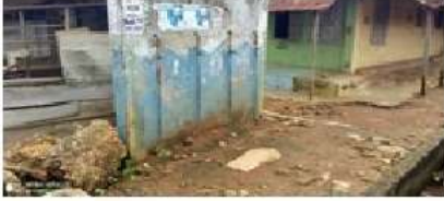
PLATE 1: ABADONED MDGs WATER PROJECT
