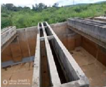
PLATE 8: MORIBOUND WATER FACILITY AT ERO DAM
