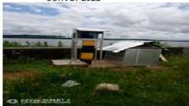
PLATE 3: ABADONED WATER FACILITY AT ERO DAM
