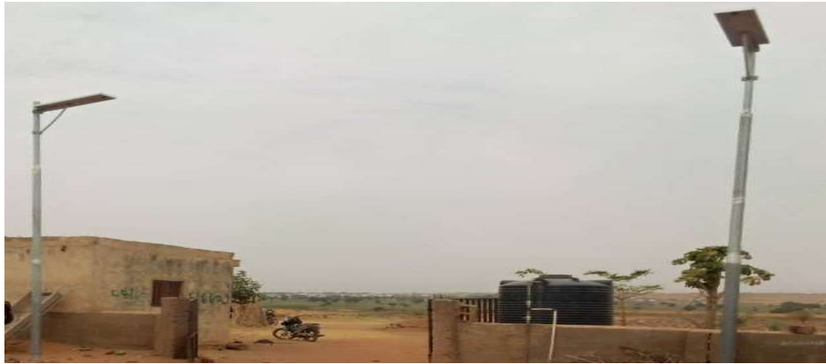
Plate 2 Solar Lightening Facilities at Kurfi Cemetery, Sokoto
