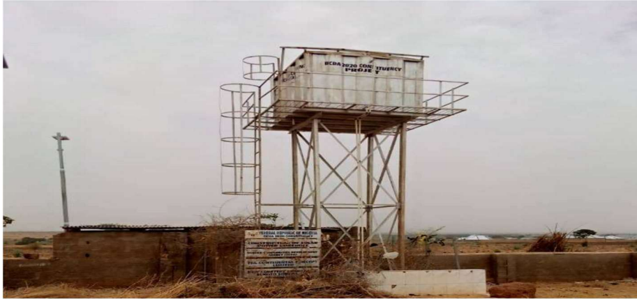
Plate 1 Water Facilities at Kurfi Cemetery, Sokoto
