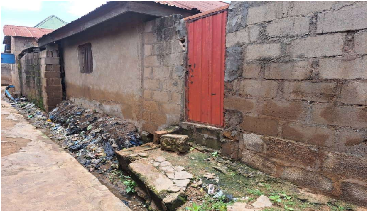
Plate 2c Condition of Drainage System at Anguwan Shanu, Kaduna North
