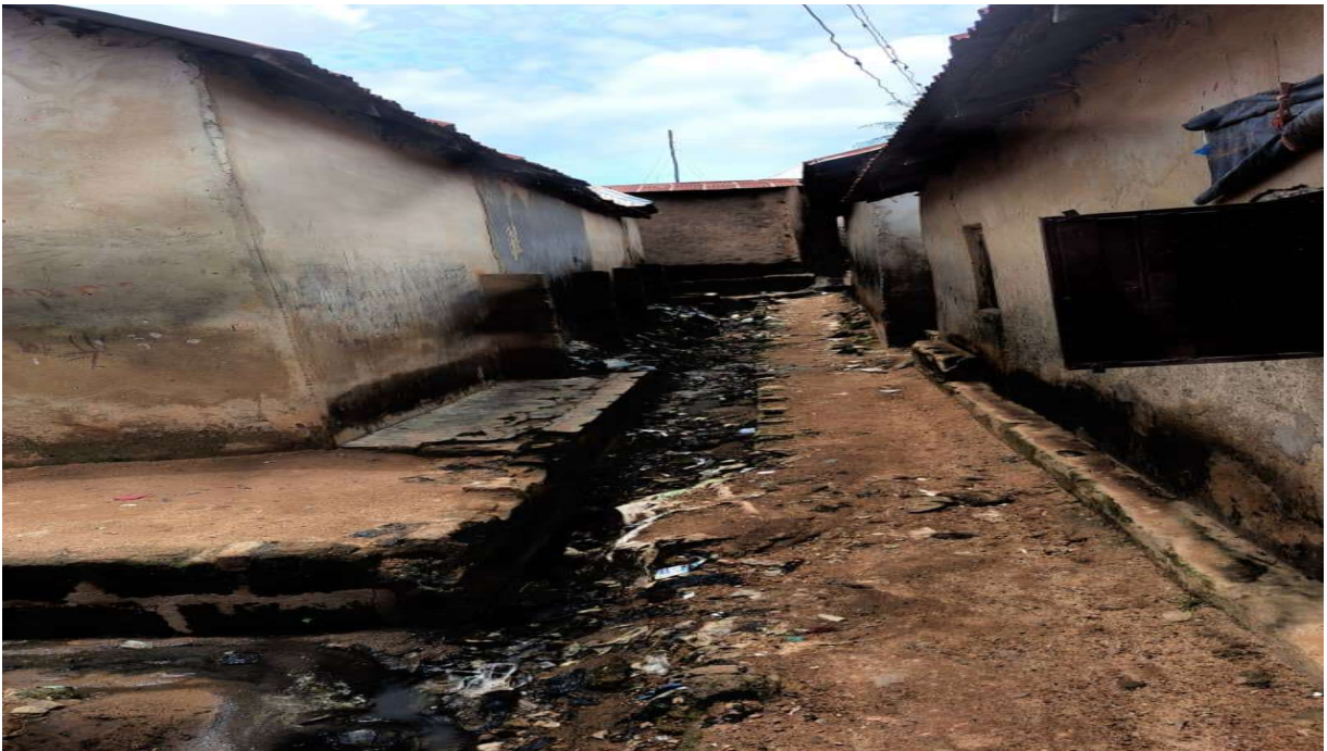
Plate 2b Lack of Good Drainage System at Anguwan Shanu, Kaduna North
