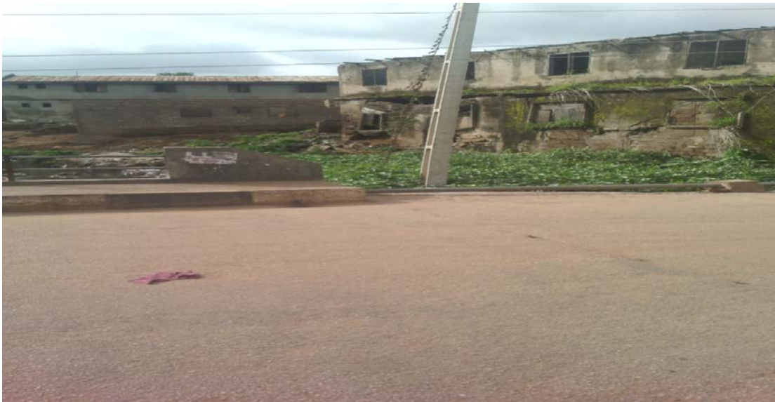
Plate 2: Vacated Building along Waterways at Oja Iya area, Ilorin. Source: Author's Field Work, 2014.
